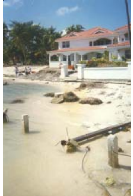
Post-Hurricane Mitch: Damaged home and seawall reaffirm the fact that development guidelines, such as setbacks are important for property protection.
